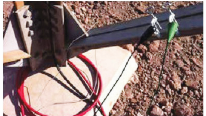
Rogowski Coil fitted around a typical tower leg. The green lead is injecting the test current and the black lead measures the voltage between the tower and the potential stake.
